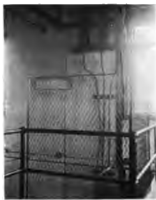
Fig. 5. Guard for 66,000 Volt Wire within reach of Platform.
